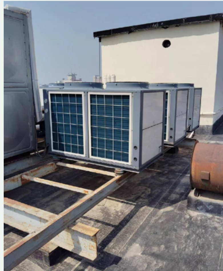
— Air Source Heat Pumps Installed at the HanTing Beijing South Station Muxiyuan Property —
